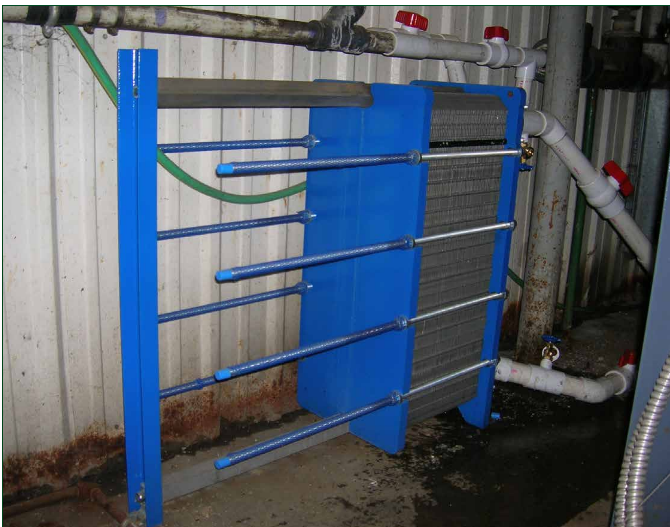
Wastewater heat exchanger at Bald Hill hatchery reduces the energy needed to heat incoming water by capturing heat from the wastewater and using it to heat the new incoming water.
